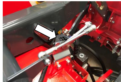
Angle sensor hoist
